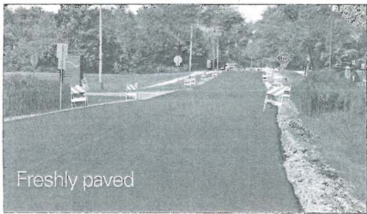
Freshly paved The project to resurface Highridge Road was nearly completed last week when workers paved the asphalt surface of the road, which is located just north of Willowbrook High School. The project included the milling and resurfacing of Highridge from Ardmore Avenue to the village's west limits. The photo, taken Saturday, shows a westward view of the newly resurfaced road. Members of Villa Park's public works department stated at recent village board meetings that the road would be resurfaced before Aug. 17—the first day of Willowbrook's 2016-17 school year. According to information in Villa Park's capital improvement program, the overall project to resurface Highridge Road carried an estimated cost of $436,000. Villa Park Village Manager Rich Keehner stated at a recent board meeting the project came in under budget. A federal grant reportedly covered approximately half of the project's cost.
